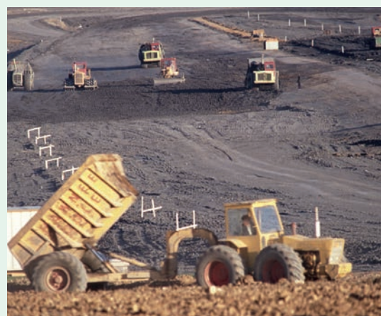
Reservoir slogs: Hard work spreading and compacting clay to line Rutland Water.
